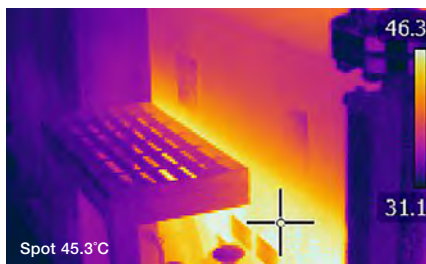
Fig. 9—Low operating fluid level in reservoir.
